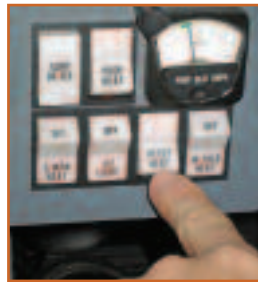
Training in how to routinely get the correct results you want from today's complex panel is an area Dick Rochfort refers to as "buttonology." This is particularly important when you've had new equipment installed.
